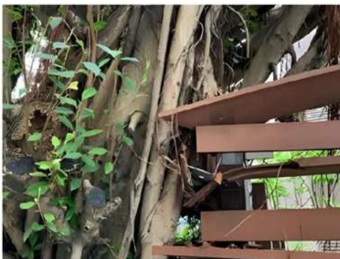
氣生根生長壓壞圍欄
